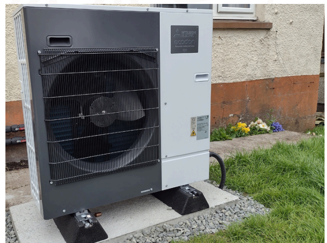
Newly installed Heat Pump at Plasterfield.
